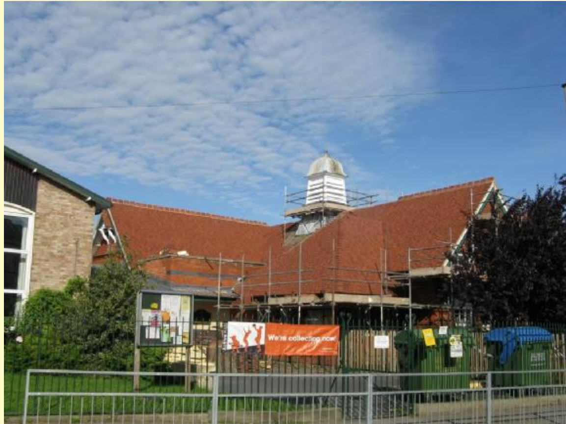
The new roof looks wonderful – a real craftsman-built job. The tower has been renovated and painted.
